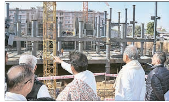
CM Ashok Gehlot, Health Minister PL Meena, Anoop Bartaria and Ravi Jain at the construction site of IPD tower on Sunday.
