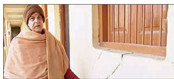
Shankaracharya Matth chief Swami Vishwapiyananda showing the cracks.
